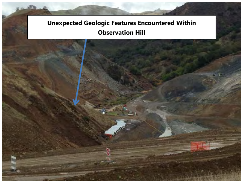
FIGURE 5 - FIELD PHOTOGRAPH OF ENCOUNTERED CONDITION
