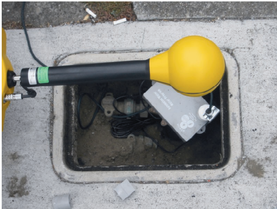
Top and bottom: Measurements at 8 inches (20 cm). The MTU has had the mounting brackets normally holding it to the bottom of the water vault concrete cover temporarily removed.
