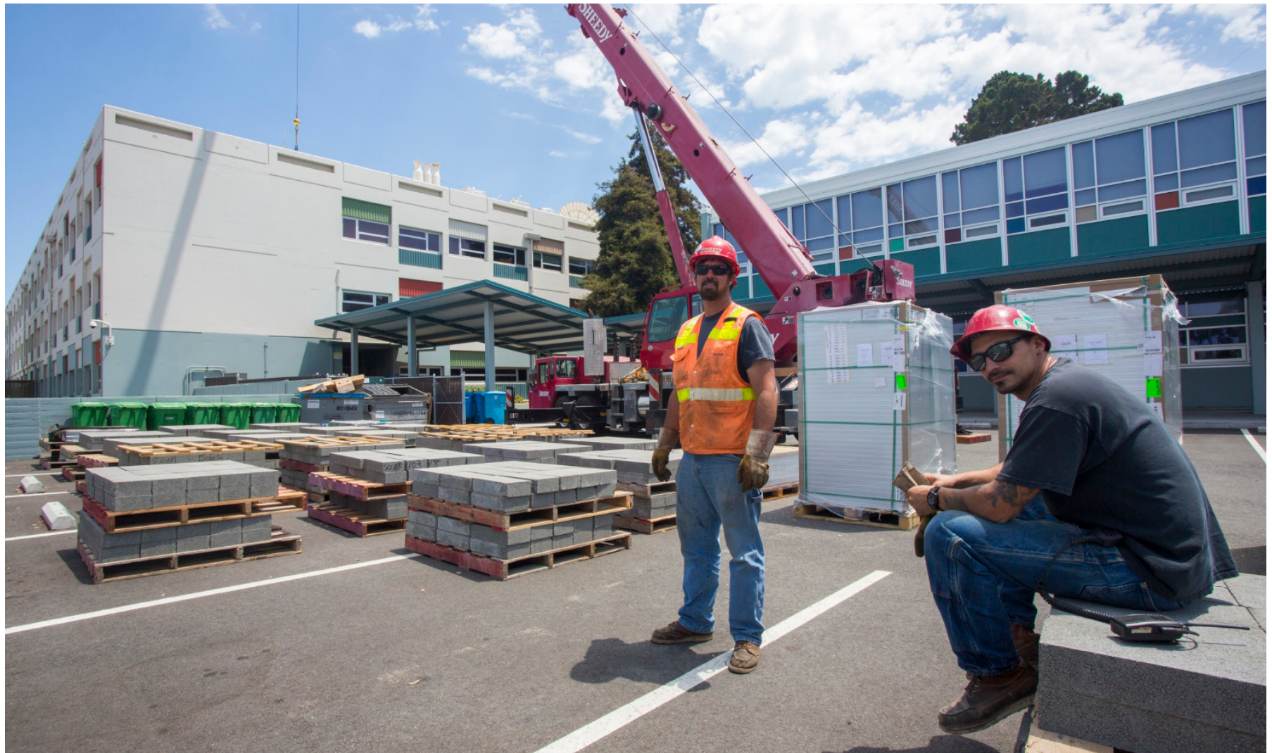
Burton High School solar installation
