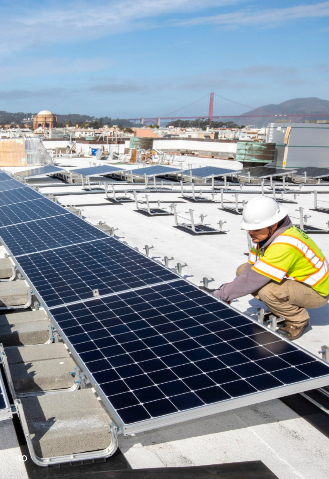
Solar panels installed at Marina Middle School
