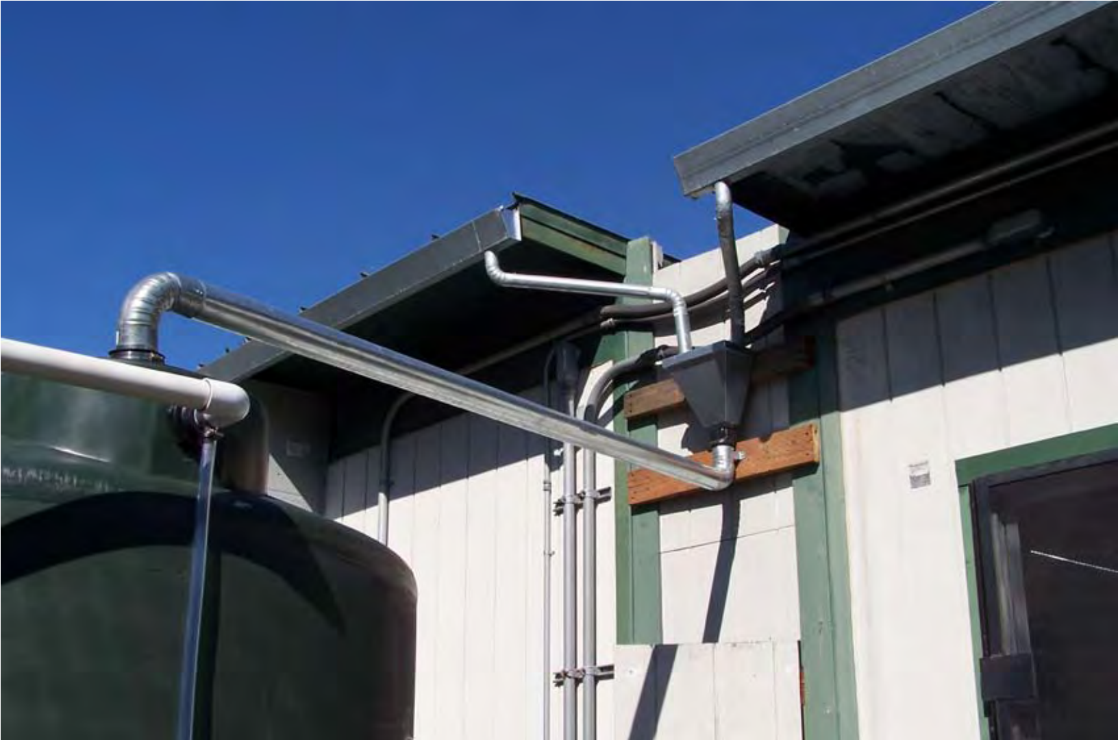
Rainwater Cistern at Alvarado Elementary School, SFUSD
