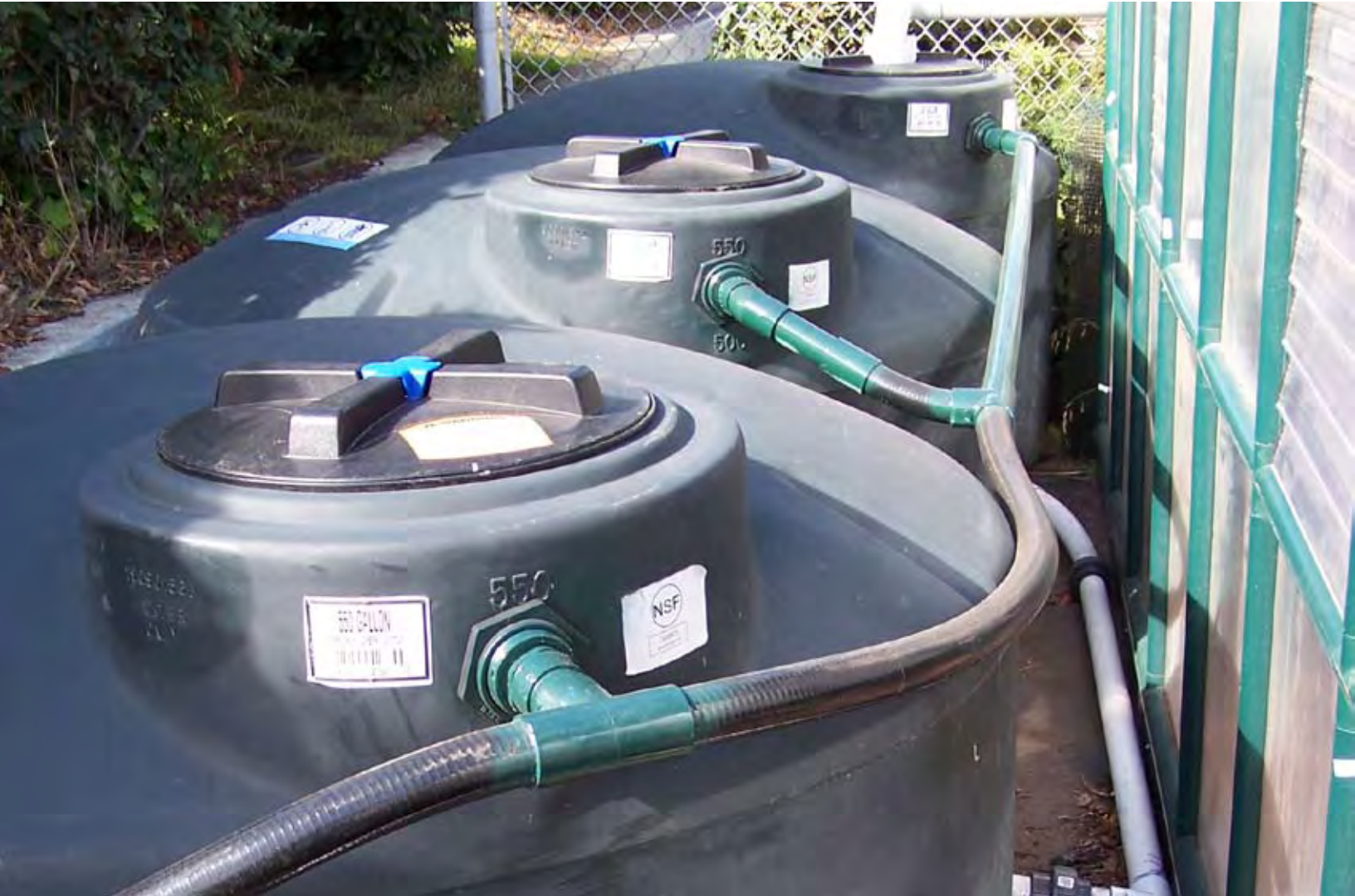
Cisterns at Miraloma Elementary School, SFUSD
