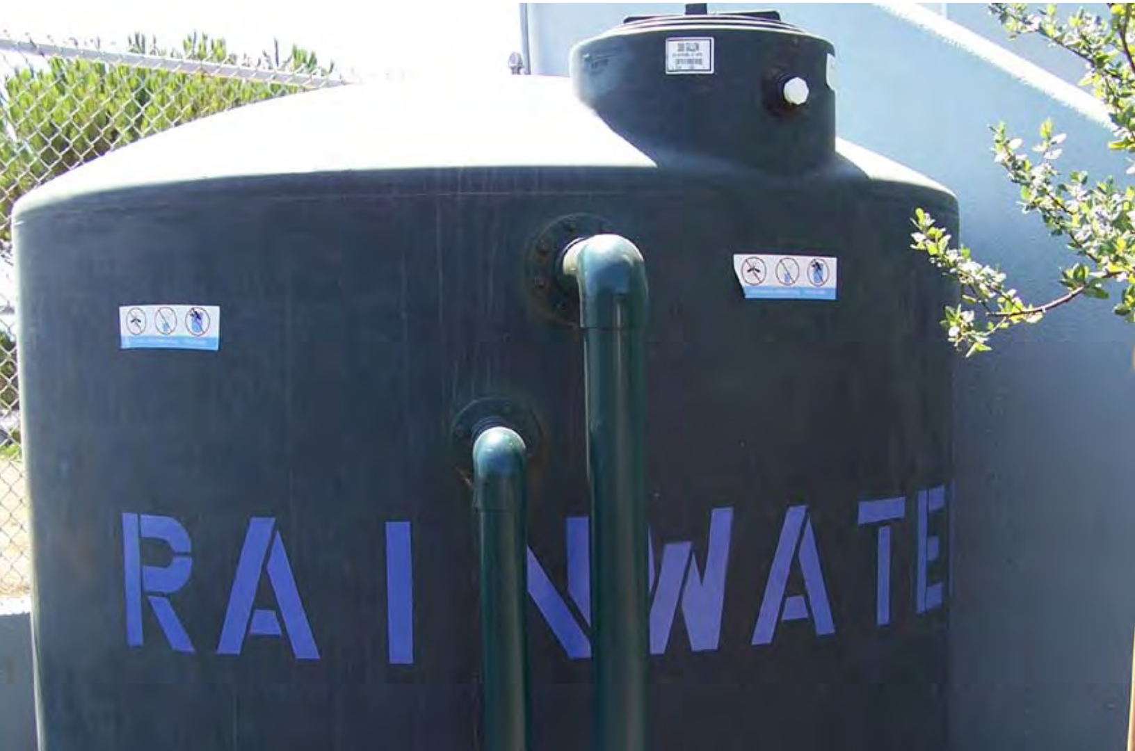
Starr King Elementary School Cistern, SFUSD
